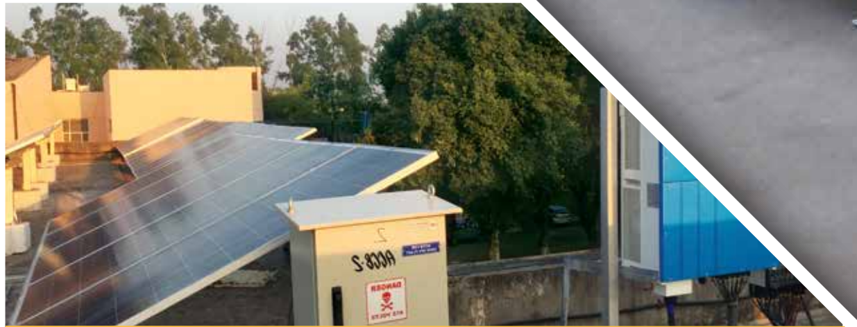
Solar Power Distribution Boards
